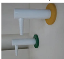
Water & Gas Tap
