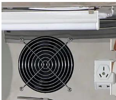
Lighting system and BOD socket
