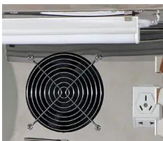
Lighting system and BOD socket
