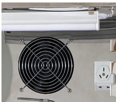
Lighting system and BOD socket
